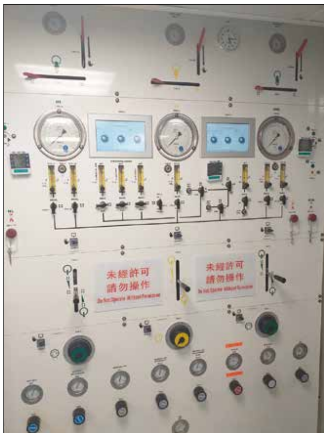
Figure 4. The manual control panel is used in case the computer control system breaks down.
